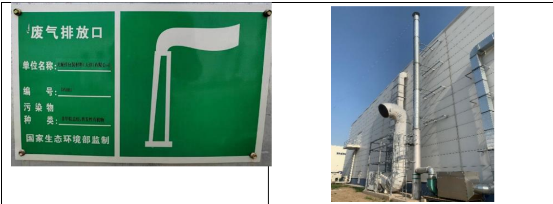
排气筒DA001 (P1)
